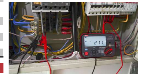
Automatic Voltage Measurement
