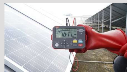
Energized device test (DC 1000V; PV)
